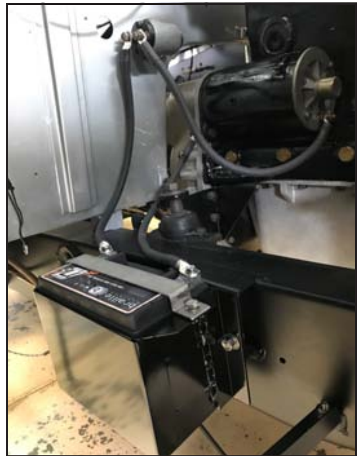
Note the custom battery cables.
